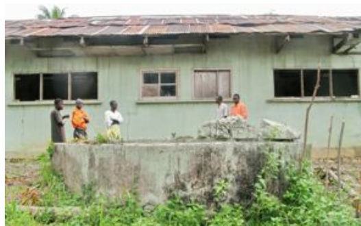
Abandoned cistern behind school.
